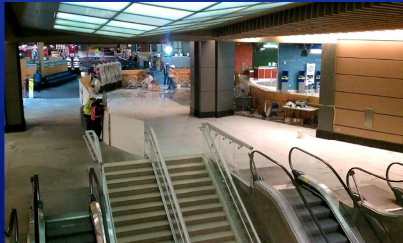
The McCarran Rent-A-Car Center's flooring upgrades will be complete by late December, in time for the New Year's Eve rush.
